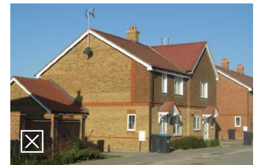
The clay hanging tile is inconsistently applied and appear to peel-away at the side. The roof tile also looks too bright in relation to the facing tile
