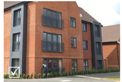
Juliet balconies can add interest to facades while providing rooms with a greater connection to the outside
