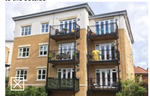
Balconies are inappropriately dominant on the façade and appear to be bolted-on
