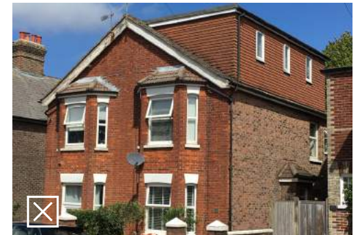
This over-sized dormer undermines the shape and symmetry of this gable frontage.
